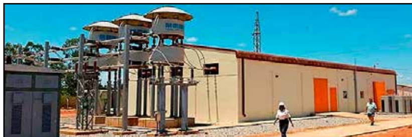
Figure 2: \pm 75\text{MVAR} , 220kV STATCOM System inside civil building (Courtesy: Montnets Rongxin Technology Group Co., Ltd)
